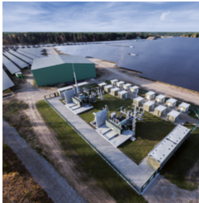
New methods for predicting the working life of components could render the generation of electricity using photovoltaic panels (here a ground-mounted plant connected to batteries in Templin) cheaper.
